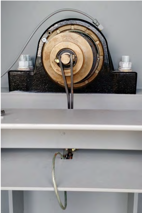
Image 3-7 – Backspin preventer installed
