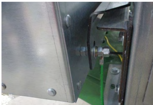
Grounding at main power box
