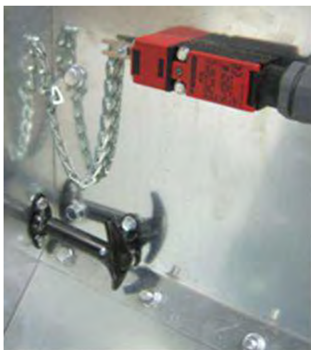
Image 4-5 – Access door switch
