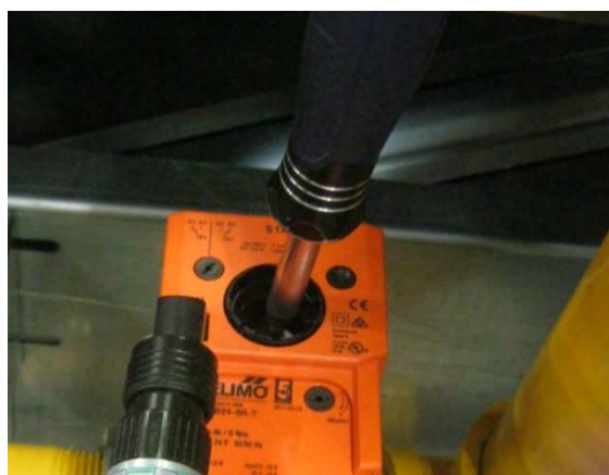
Image 8 – Setting valve to 0% open
