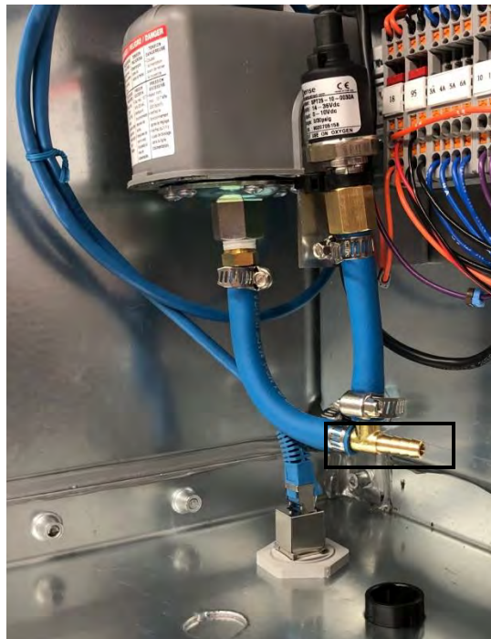
Image 4 – Air hose nozzle in power box
