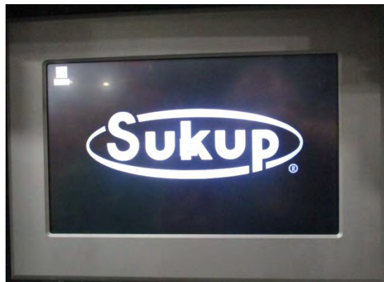
Image 5 – Control panel (N23476)
